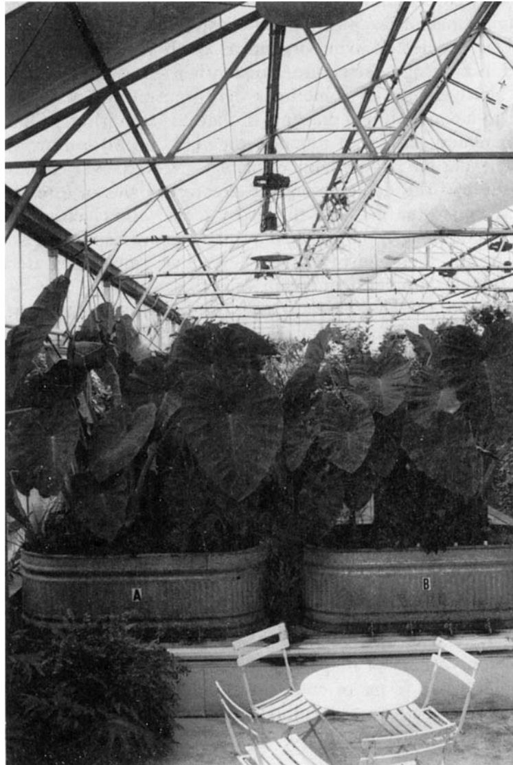
Living filters for the final polishing of the purified sewage. Photo by John Todd.
