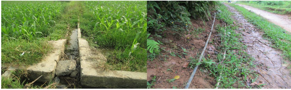
Fig. 3. Irrigation canals and water pipes in the research areas.
