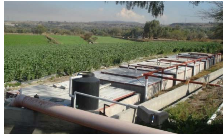
Figure 2: WWTP with quinoa crop (Acoculco, Hgo.)
