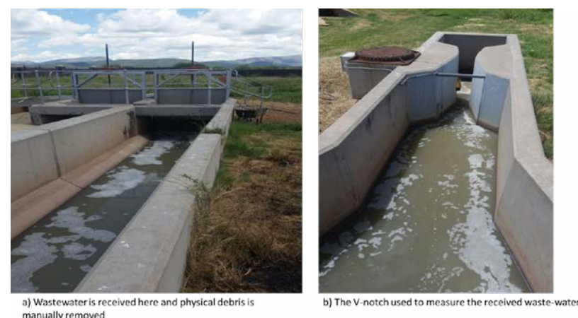
Figure 2: Physical screening of solid waste and V-notch weir at Lebowakgomo wastewater treatment plant
