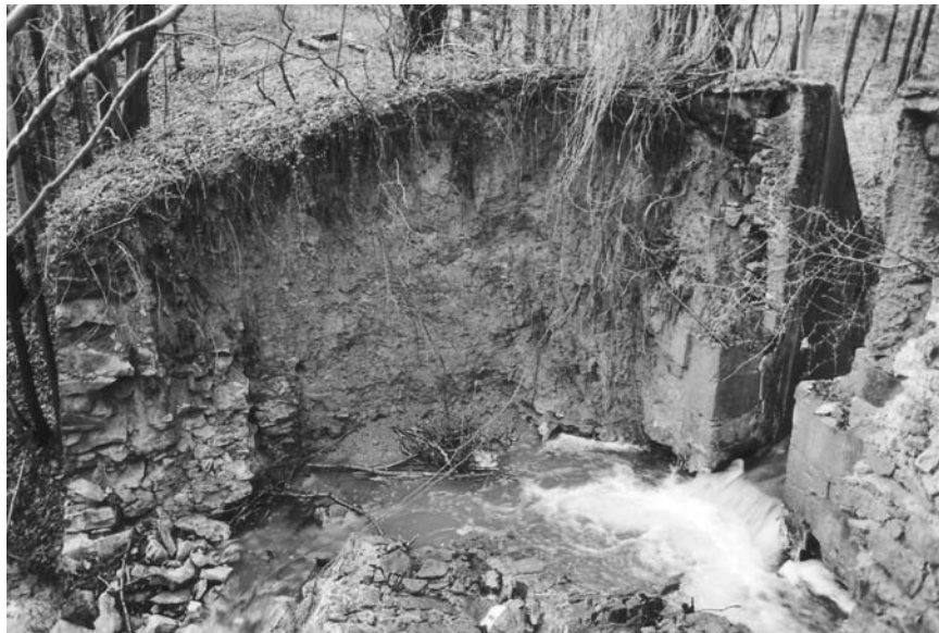
Figure 13.11 A downstream view of the eroded part that once included the discharge tunnel
