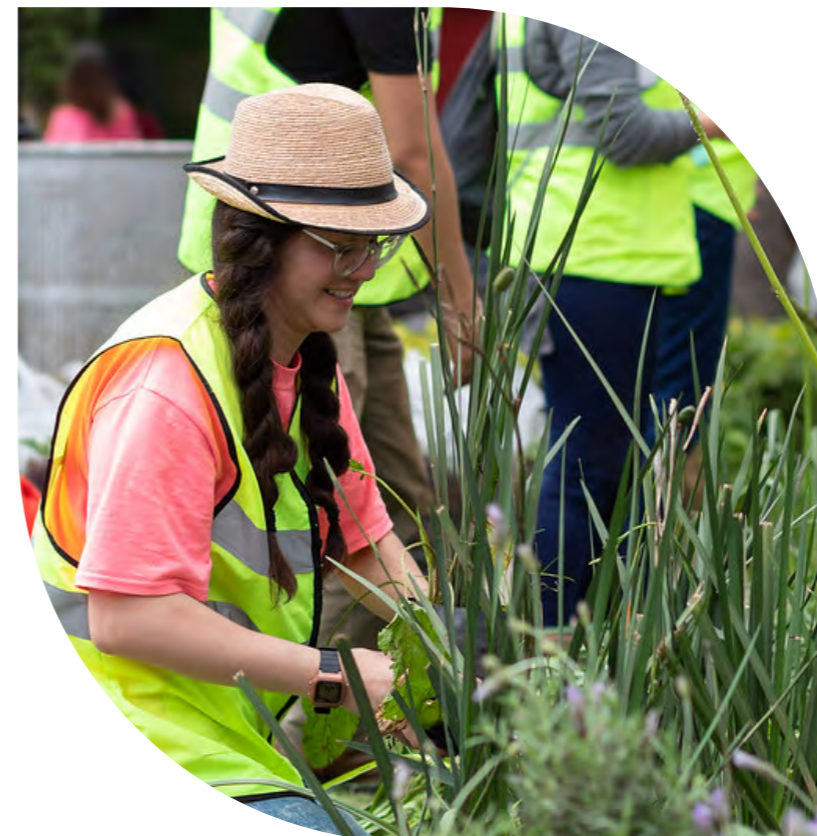
Placement of urban furniture and vegetation in Plaza Revolución and delimitation of crosswalks, August 2023. © WRI México
