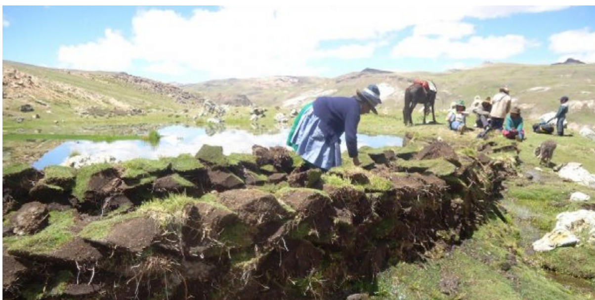
Construction of a dam in a qocha during a farmer's contest. © Helvetas Swiss Intercooperation / PACC project
