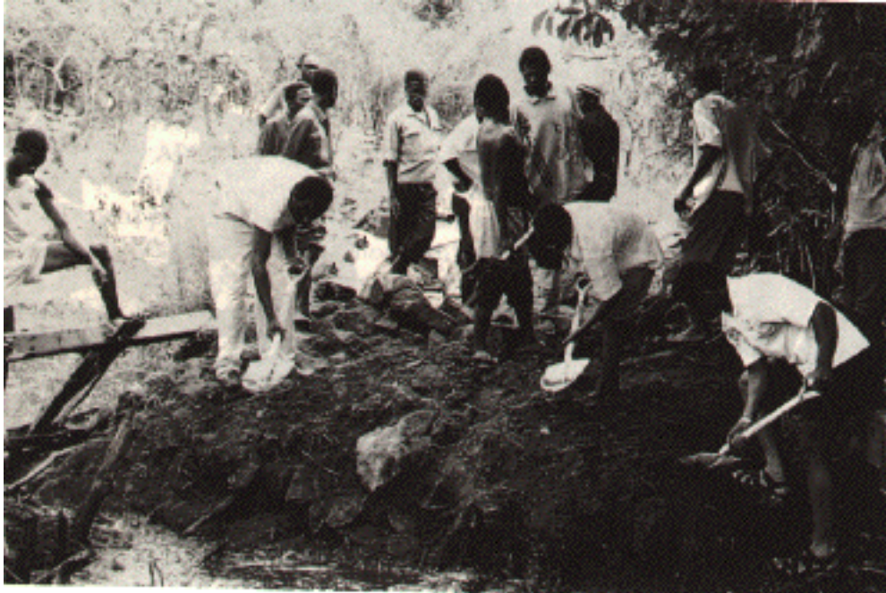
Fig. 6. Road Building by Village People Across the 3-km Wide Marshlands of Lubangule River. A total of 100 km of dirt roads have been restored
