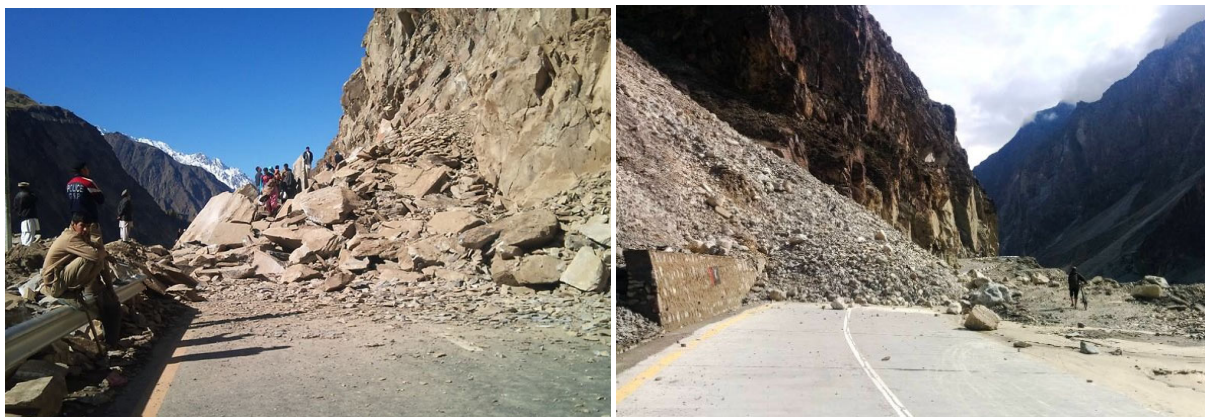
Figure 4 Geo-hazards along China-Pakistan Economic Corridor. a. Landslide on Karakoram highway (Left) (March 2016); b. Landslide on Karakoram highway (Right) (April 2016) (Source: Tayyeb Akram 2016).
