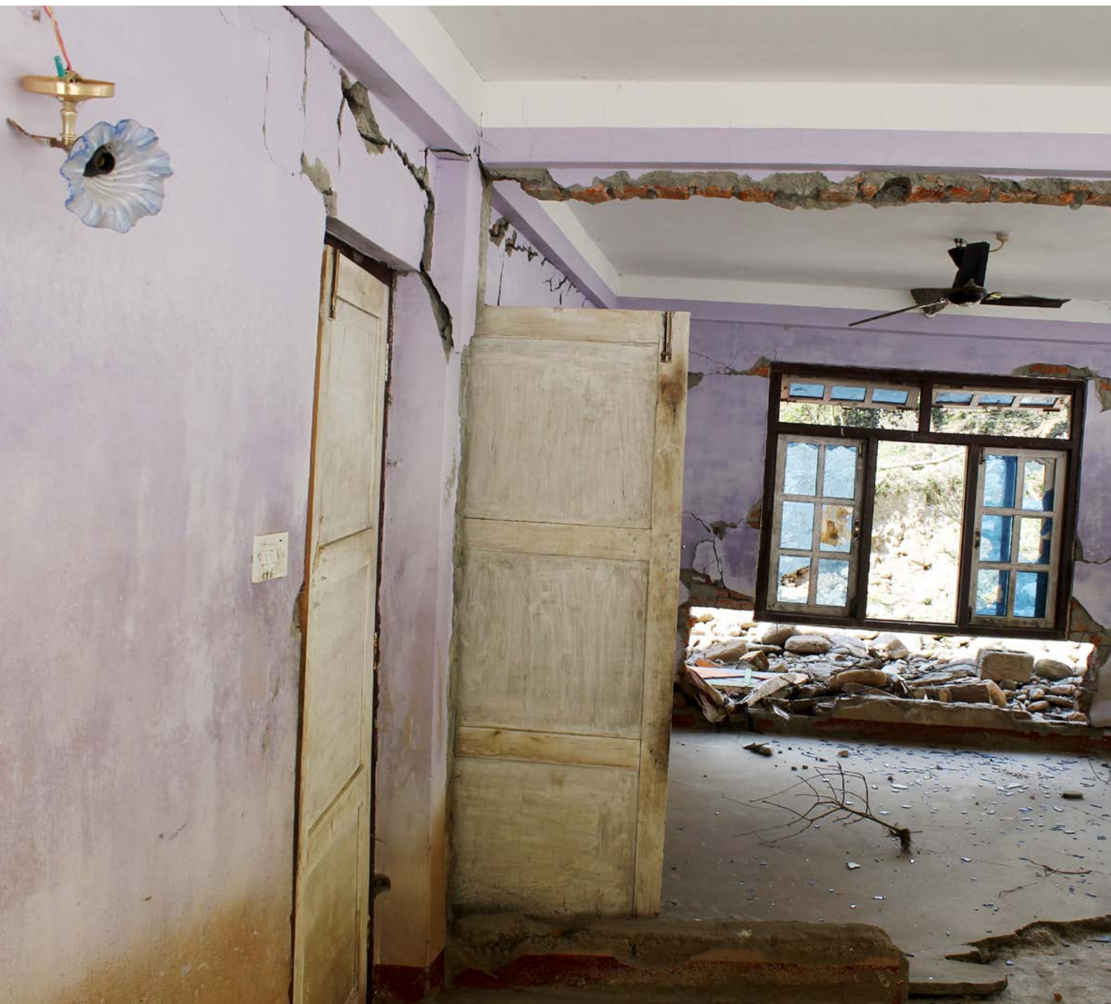
Image 17: The interior of a house that was severely damaged and abandoned after the landslide
