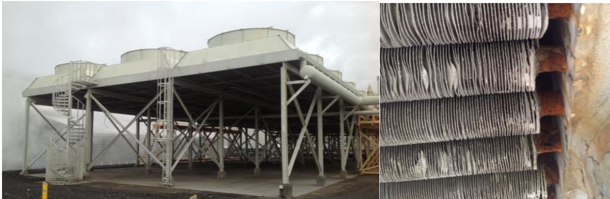
FIGURE 18: Air condensers and the leakage zone
