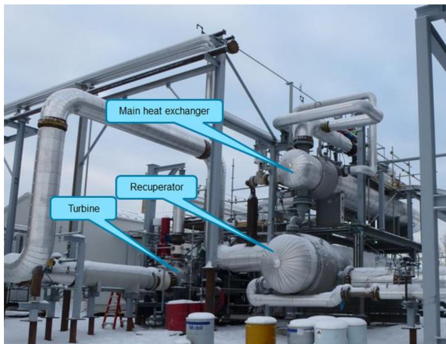
FIGURE 12: The hot end of the transcritical ORC plant in Judy Creek, Canada
