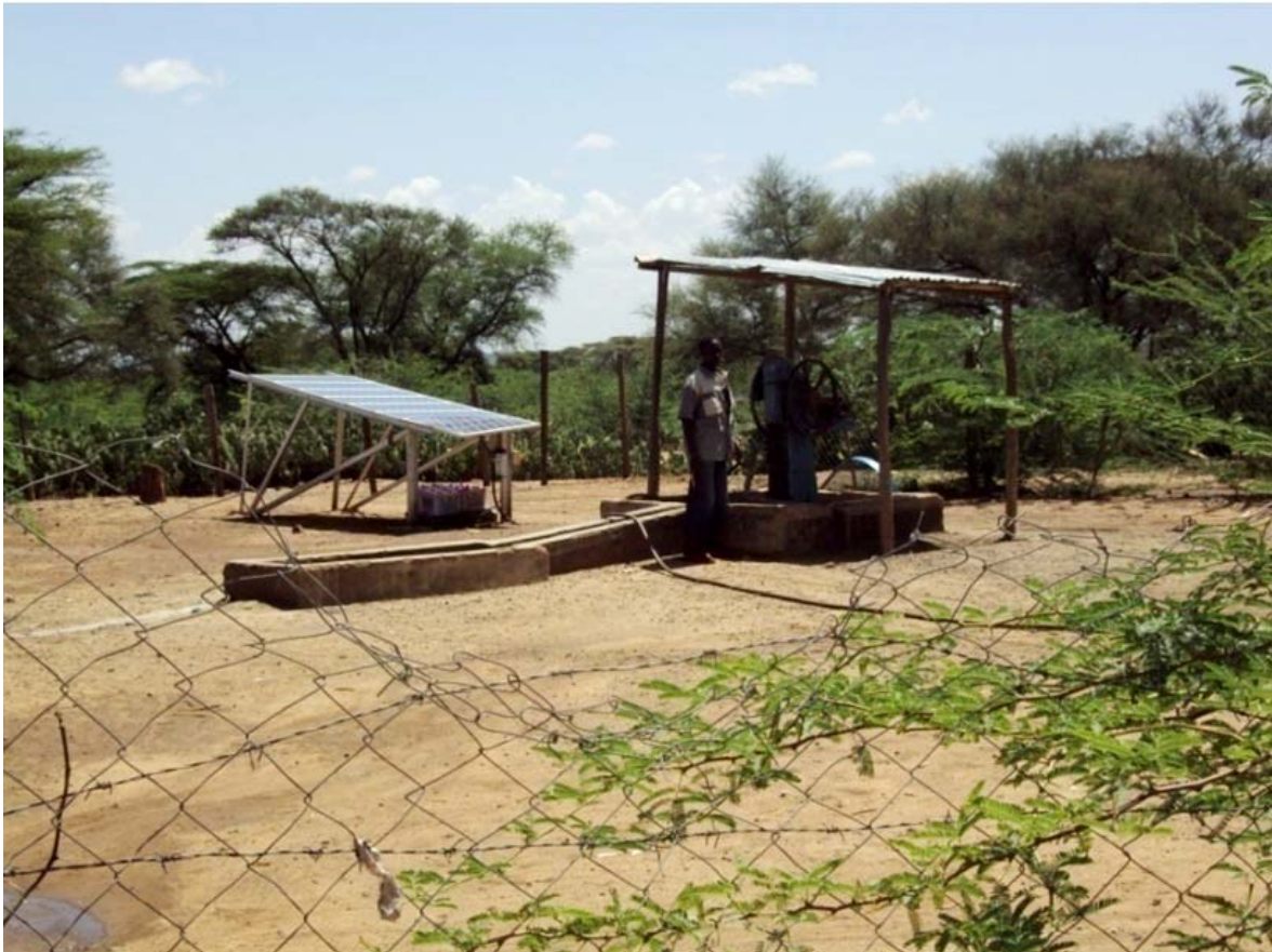
Figure 3-13: Pumping of borehole water using solar energy at Kampi ya Turkana (Marigat)
