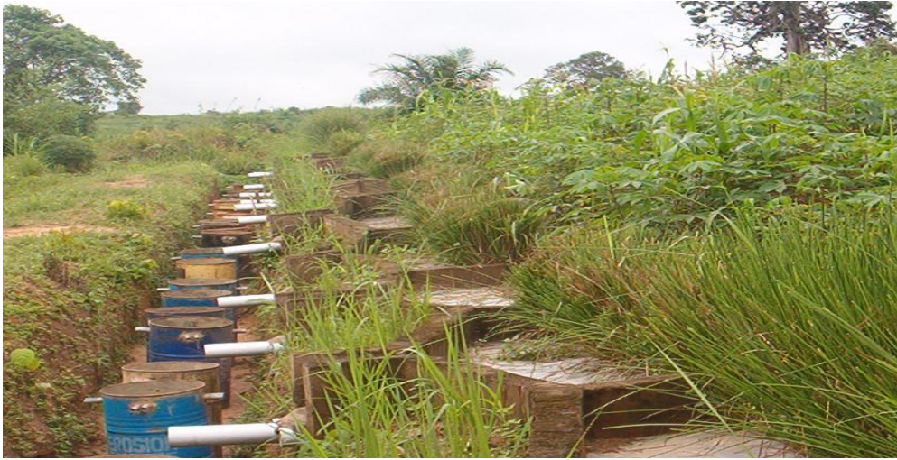
Figure 4: Sedimentation drums installed in the ground in a trench dug at the lower end (down slope) of the erosion plot, with vetiver buffer serving as erosion control measure.
