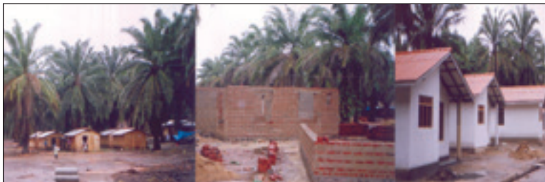
Preparing the land for housing construction (left), partially constructed houses (middle) and completed houses (right).
