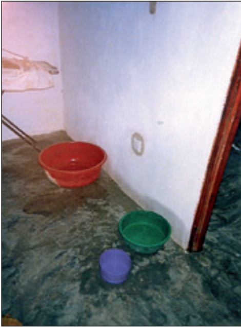
Picture 12: Water leaking from the roof of a house at Katupolwaththa Occupants have placed small buckets to collect rainwater to prevent further dampness
