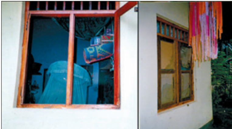
Picture 20: Windows of a damaged house as a result of physical conflict between old villagers and Katupolwaththa settlers Damaged glass window (left) and a damaged window temporarily covered with cardboard (right).
